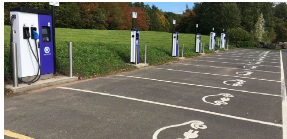
Electric Car Charging Station, Chicago (USA)
