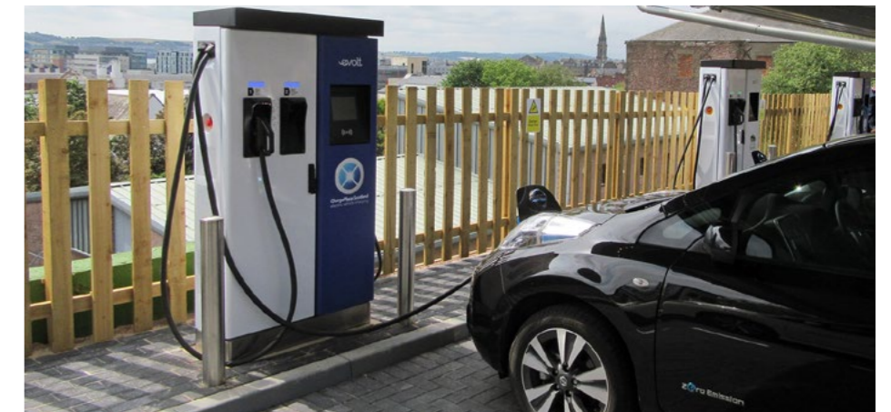
Electric Car Charging Station, Dundee (UK)
