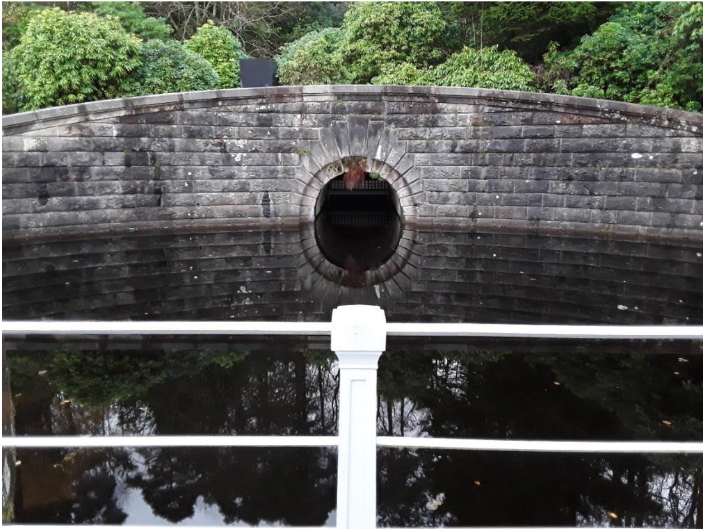
The strong, highly formal architecture of the conduit exit presented in a designed, directed view.
